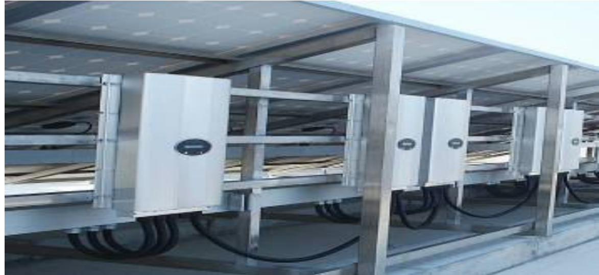
Tainan Plant 21.6KW PV System (w/Delta's Inverters)
